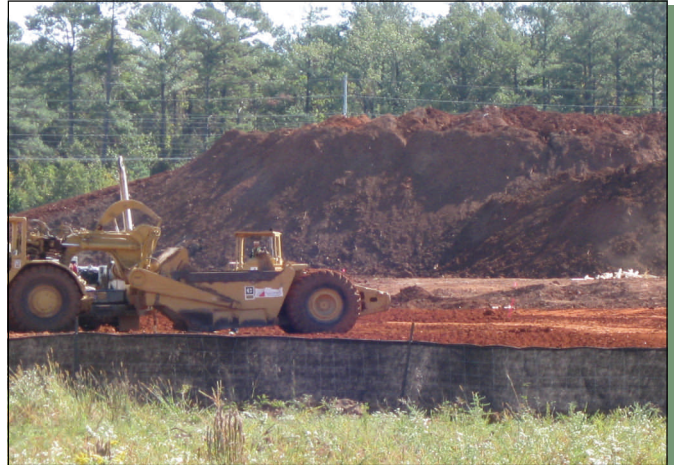
Polyplex's new site, located in Mallard Fox Creek Industrial Park; Thank you to the City of Decatur & the Morgan County Commission for helping clear the way for construction to begin
